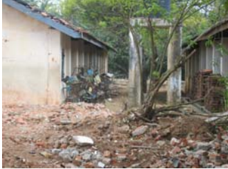
Galle School after tsunami
